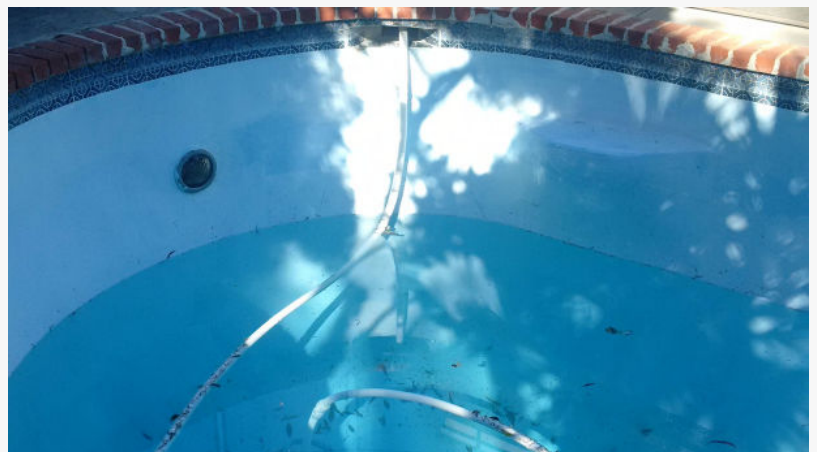
Empty Pool From A Pool Leak
